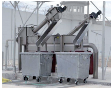
Prison wastewater treatment plant
