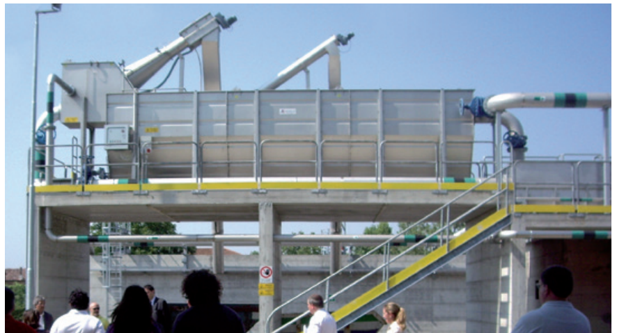
Municipal wastewater treatment plant
