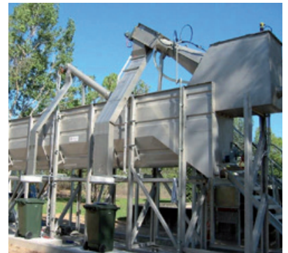
Municipal wastewater treatment plant
