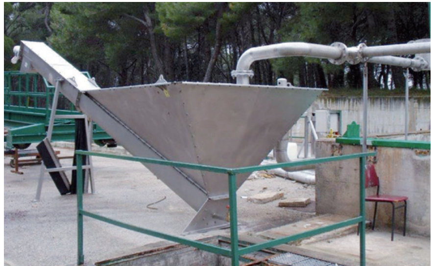
Municipal wastewater treatment plant
