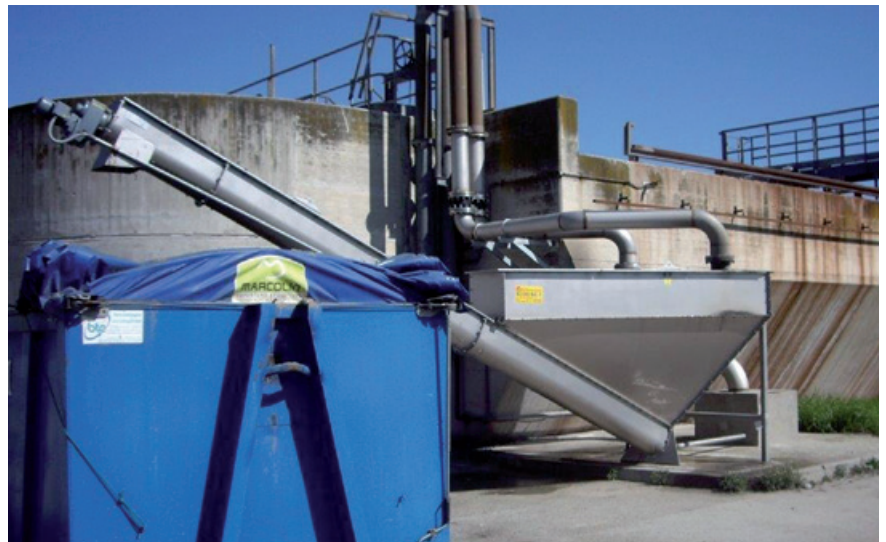
Municipal wastewater treatment plant
