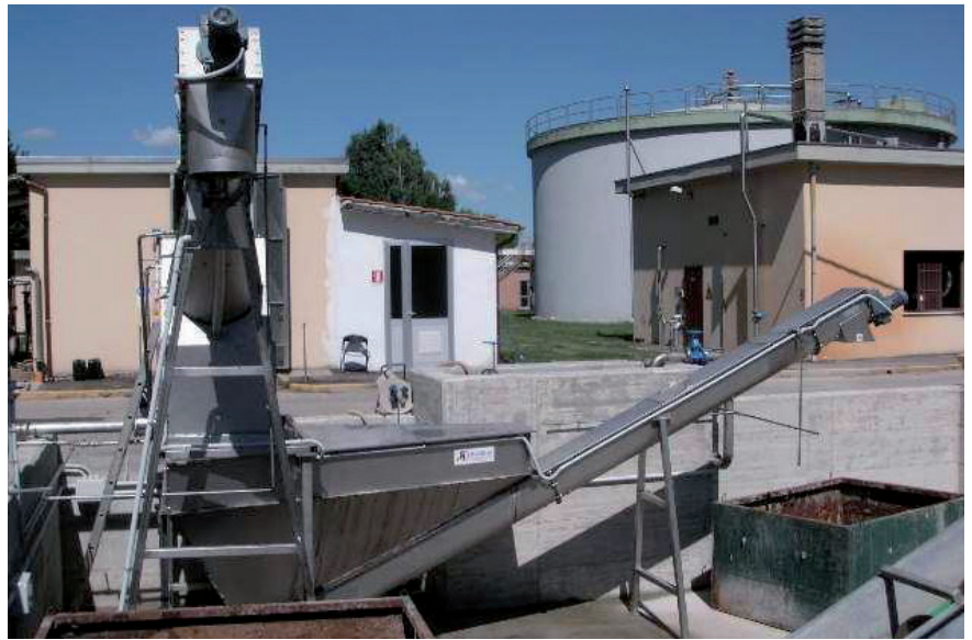
Combined System M2 municipal wastewater treatment plant application
